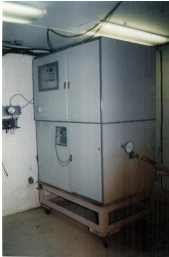
FIGURE 4. PHOSPHOLYZER Cabinet inside Analyzer Building
