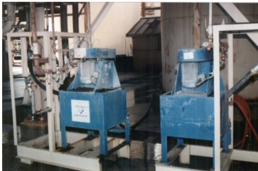
FIGURE 8. Illustration of Primary Sampling Unit with Pumps for Transfer to the Analyzer
